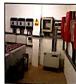
POWER BACKUP FOR ALL COMMON FACILITIES
